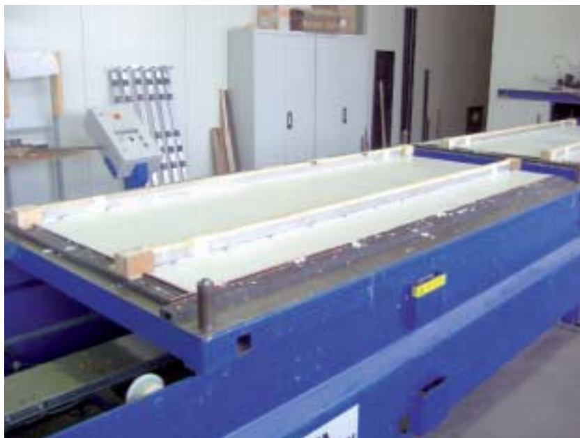
Fig. 6 Concreted slab, with the cross-beams that fix the embedded parts in position.
