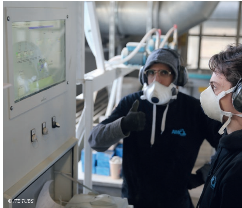
The complete control system and the power unit were supplied by Bikotronic. This allows the concrete formulation to be digitally controlled and dynamically adjusted.
